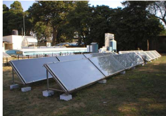
Figure 7: Solar air heating unit installed at SPRERI
