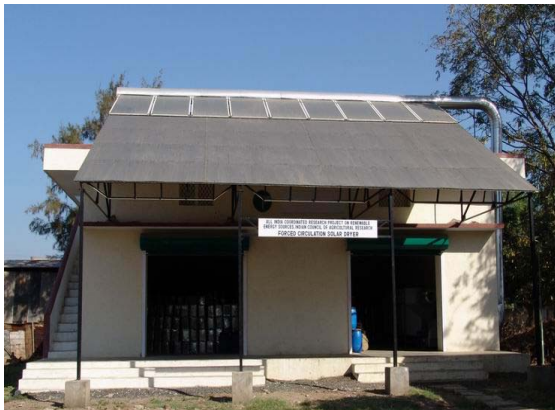
Figure 5: Glazed and unglazed solar air heaters at GSFDC
