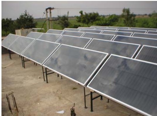
Figure 2: Packed bed solar air heaters installed at Ahmedabad
