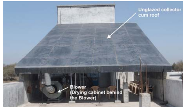
Figure 4 Unglazed solar air heaters installed at Village: Itola
