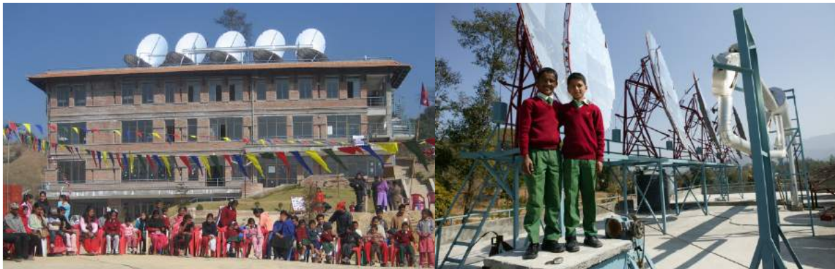
Solar steam installation on the roof of the Vajra Academy
